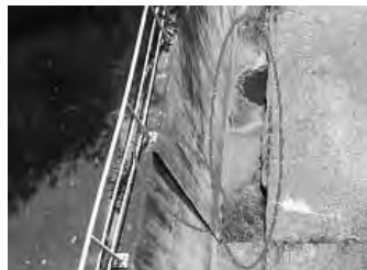
擁壁護岸の沈下・傾倒
